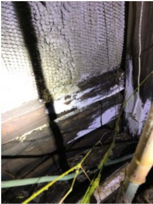
SUSPECT MOLD/FUNGAL GROWTH
