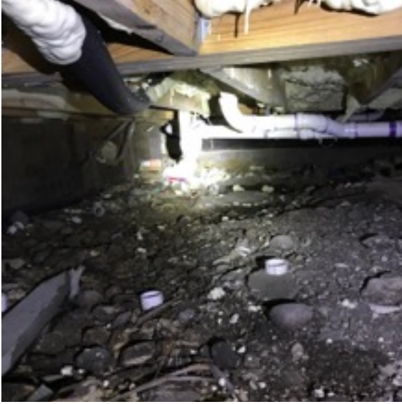
EXCESS MOISTURE AT BACK CORNER
