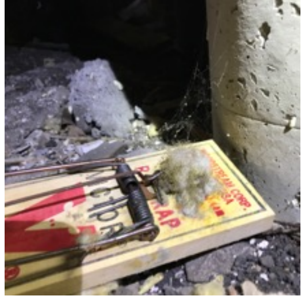
MOLD/FUNGAL GROWTH AT TRAPS
